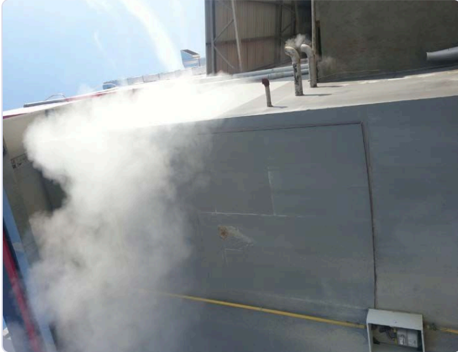
Plant 2 roof vents on steam traps: a steam plume.
