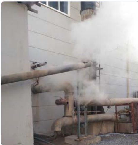
Plant 1 before the change: flash steam escaping at the condensate pipework, the steam the closed cycle now keeps in the system.
